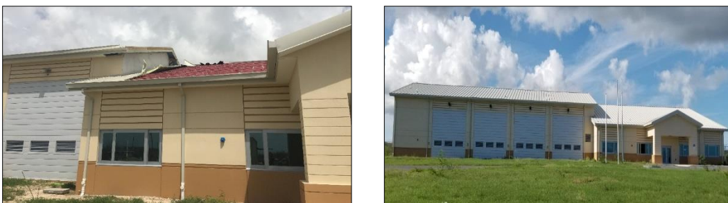
The damaged roof of the new HERA ARFF building has been completely replaced.
