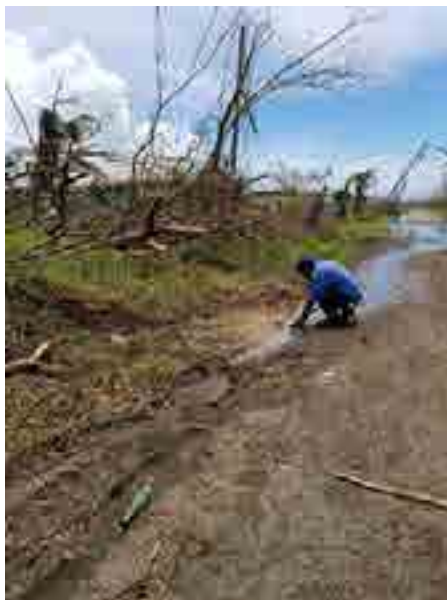
Water leak on St. Croix Source: WAPA
