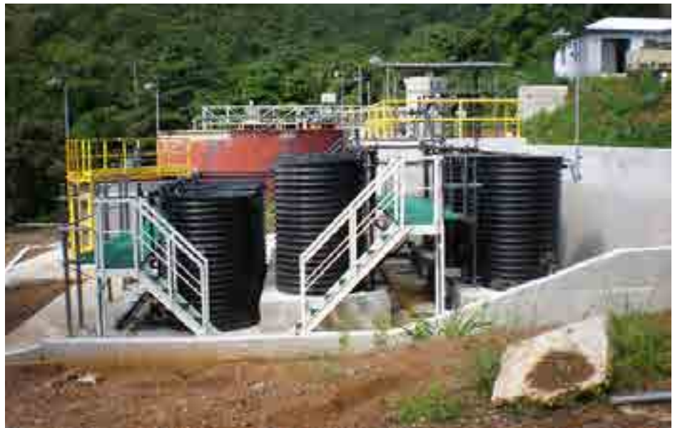
Bordeaux Wastewater Treatment Plant. Source: VIWMA
