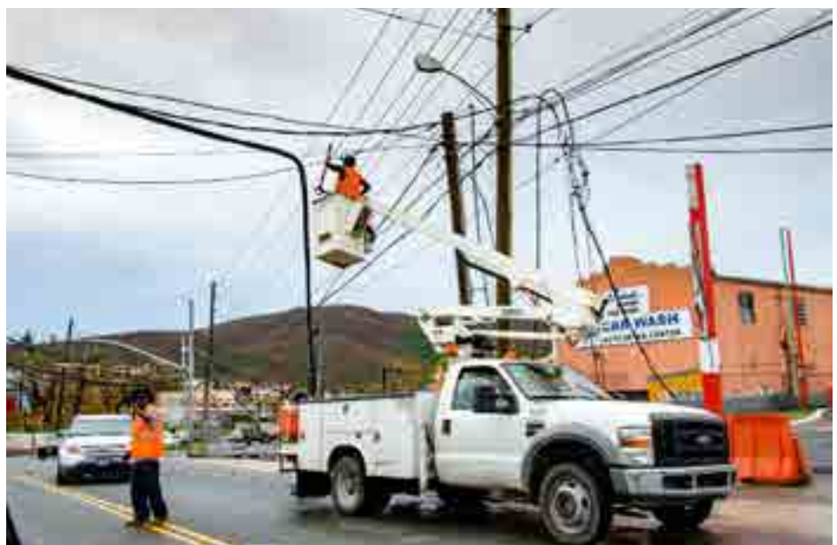
Aerial cables attached to WAPA poles
